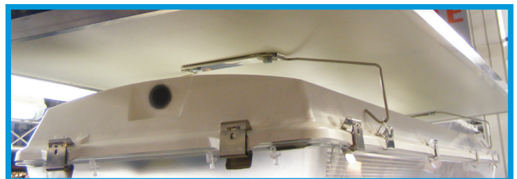
1.25" Between Ceiling and Enclosure
